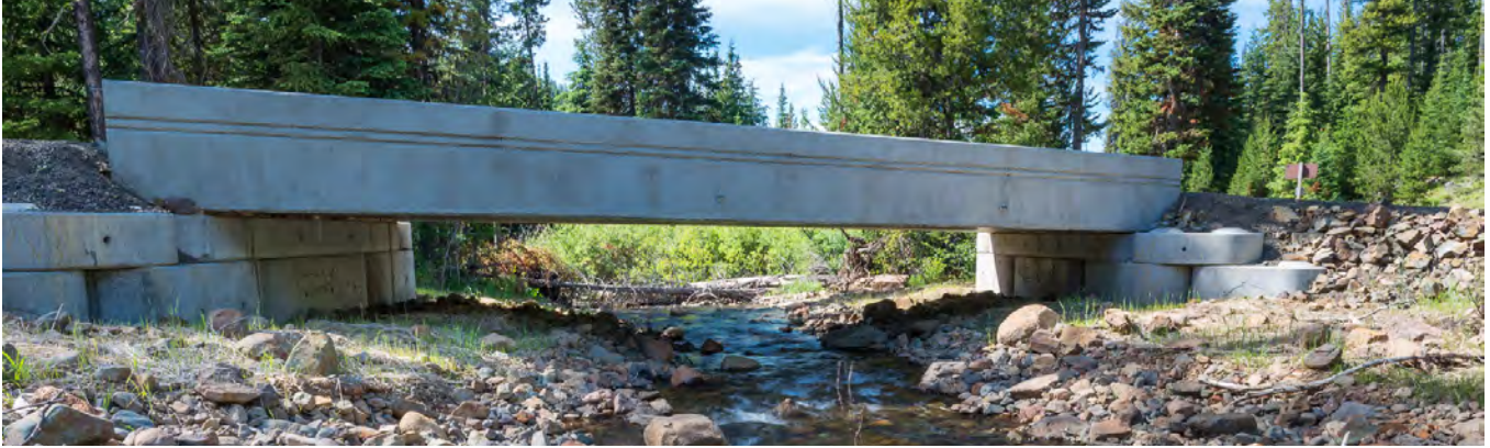
The Lick Creek culvert was replaced with a 40-foot-span concrete bridge, eliminating spawning and rearing habitat barriers for steelhead, spring Chinook salmon, bull trout and Pacific lamprey.
